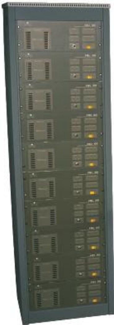
Rack with 10 units EMU-100 installed
